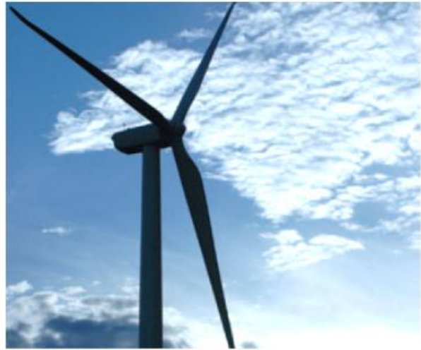
The 99 turbines at our Spearville, Kan., Wind Energy Facility produce enough environmentally friendly, emission-free electricity to supply nearly 49,000 homes annually.
